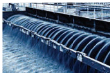
Waste Water Treatment
